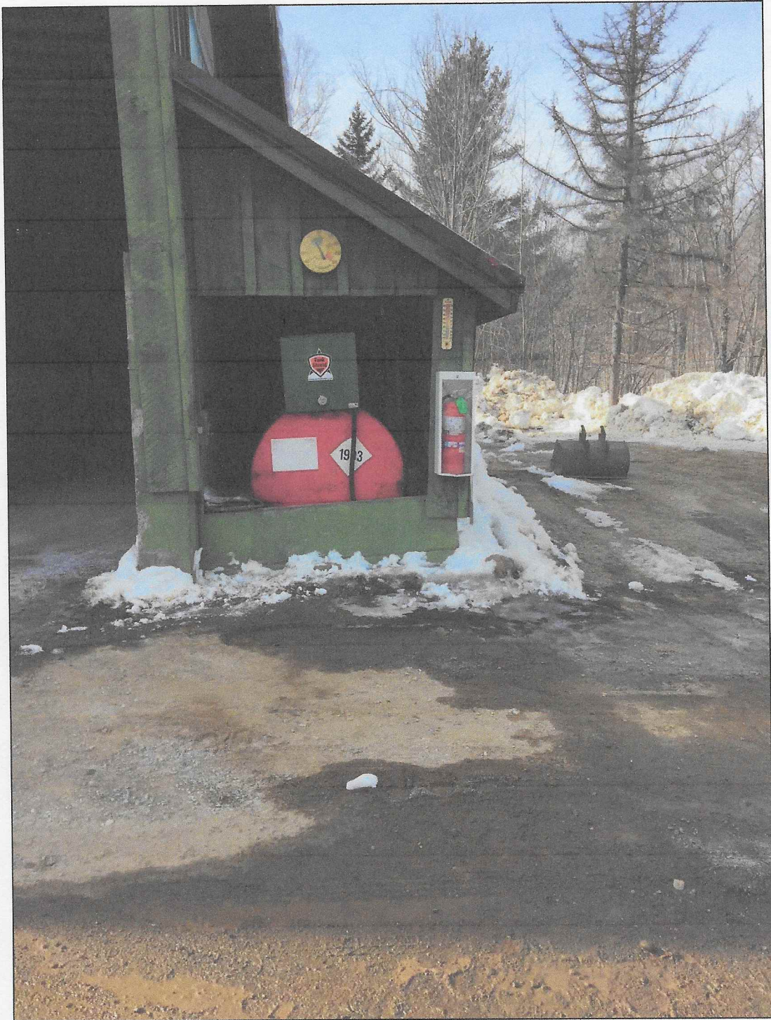
Photograph 1: Diesel AST/Spill Origin.
