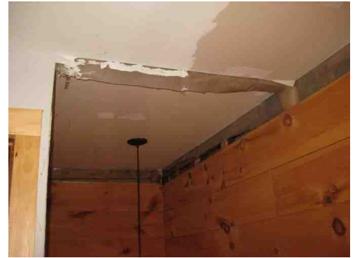
Unfinished over stairwell
