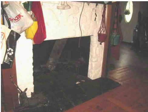
Fireplace unsound/sloping flr
