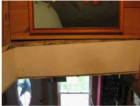
Evidence of settlement
