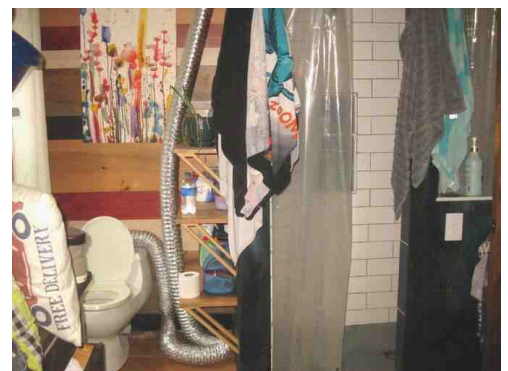
Bath repairs needed
