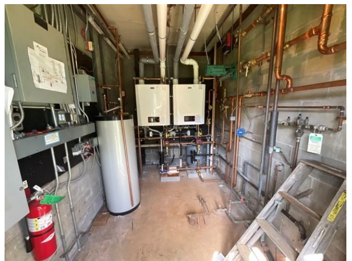
12 - PRIMARY MECHANICAL ROOM
