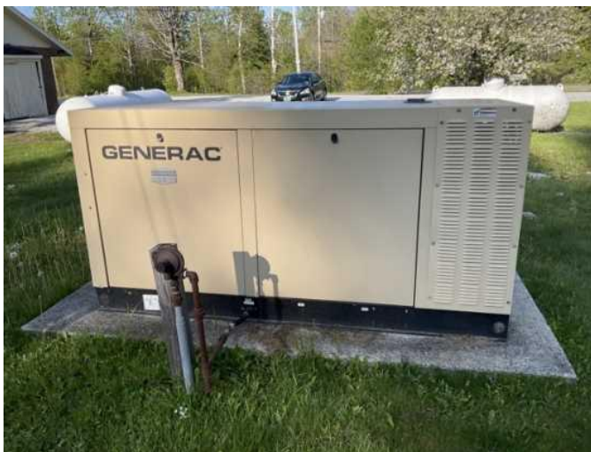
21 - PROPANE EMERGENCY GENERATOR
