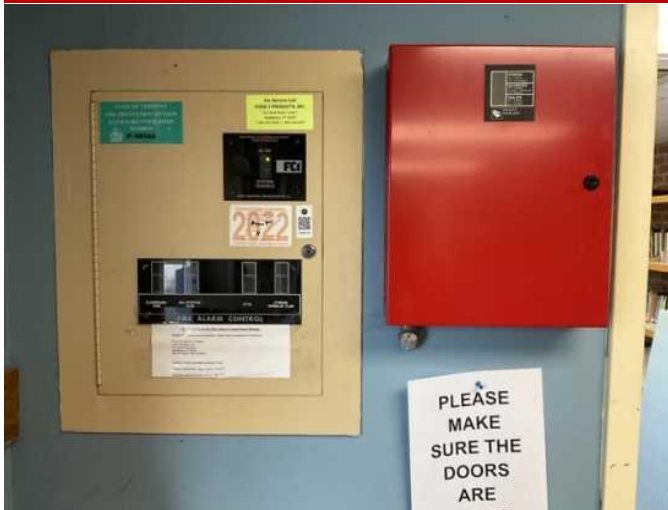
19 - FIRE ALARM SYSTEM
