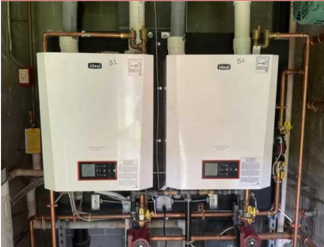
13 - HOT WATER BOILERS
