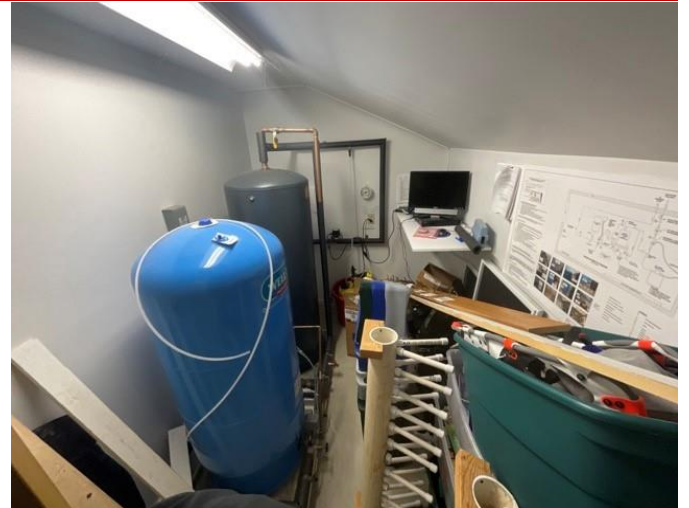
14 - INCOMING WATER FROM WELL
